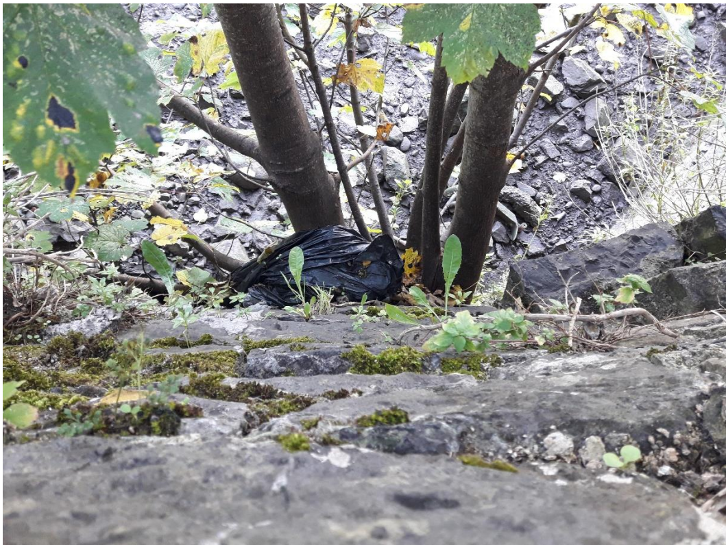
Photograph 7: As they expand, the roots of tree 12 will push and weaken the structural integrity of the wall.
