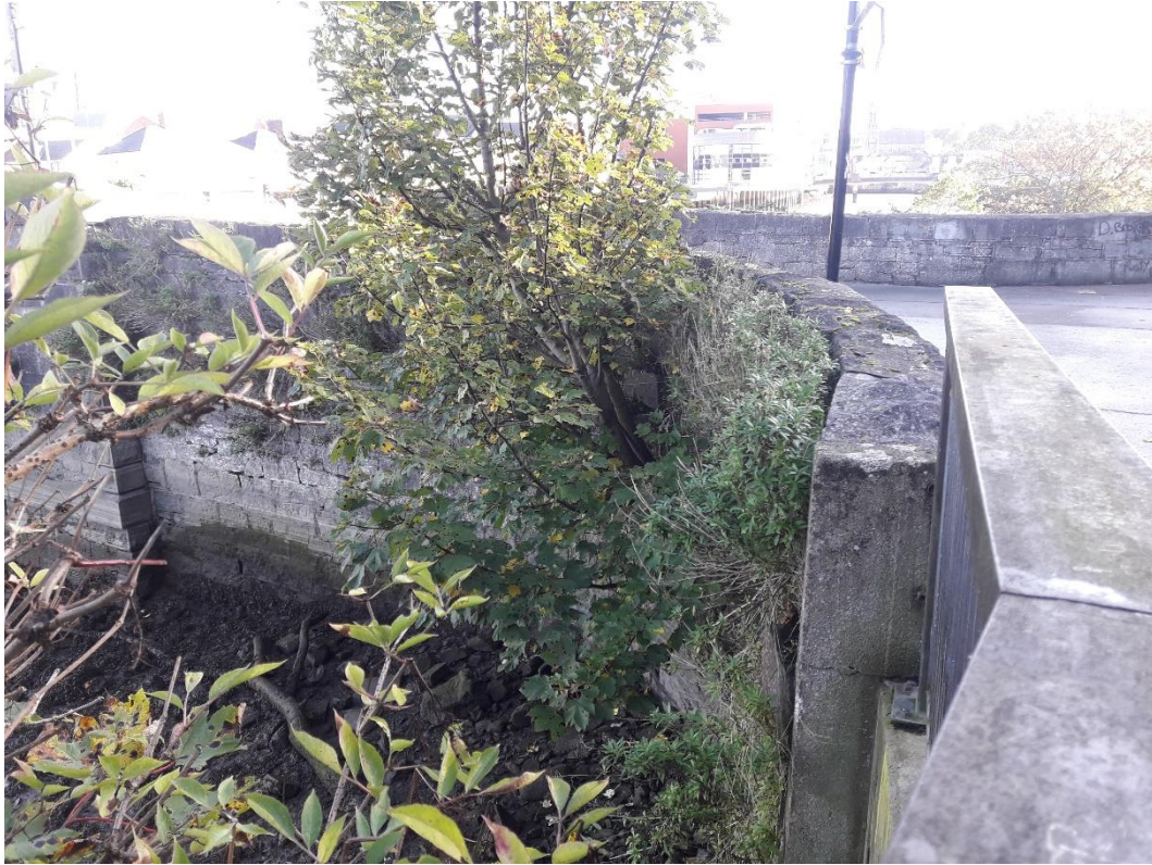
Photograph 6: Tree 12, growing from the wall of the bridge.
